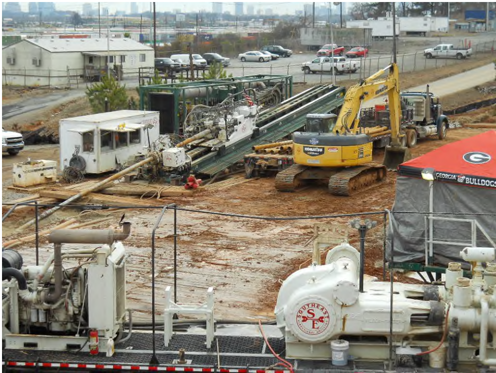
This final picture depicts the lay down area for a large diameter HDD in an urban environment.
